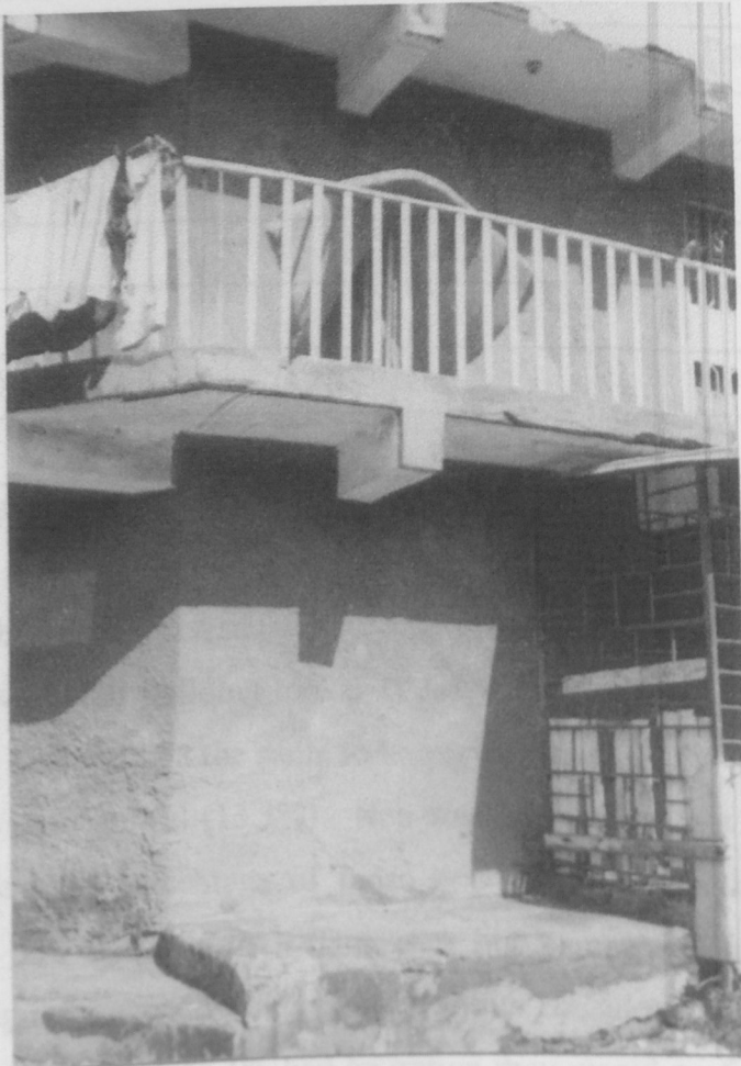
Plate4: Cracks which appears at the ground floor and the first floor as shown have been plastered, hence the non-uniformity of the rendering. As told this cracks are always plastered after every 3 months, because they keep on recurring.
