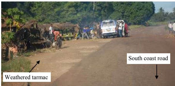
Bus stop at Mwangwei Junction (gate 01, Fig. 5.5 a) illustrating weathered tarmac exposing road murrum.
