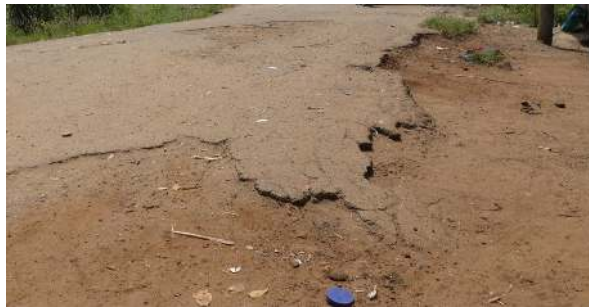
Side paved road intersection at Bwiti Junction (gate 07, Fig. 5.4) illustrating weathered tarmac exposing road murrum.
