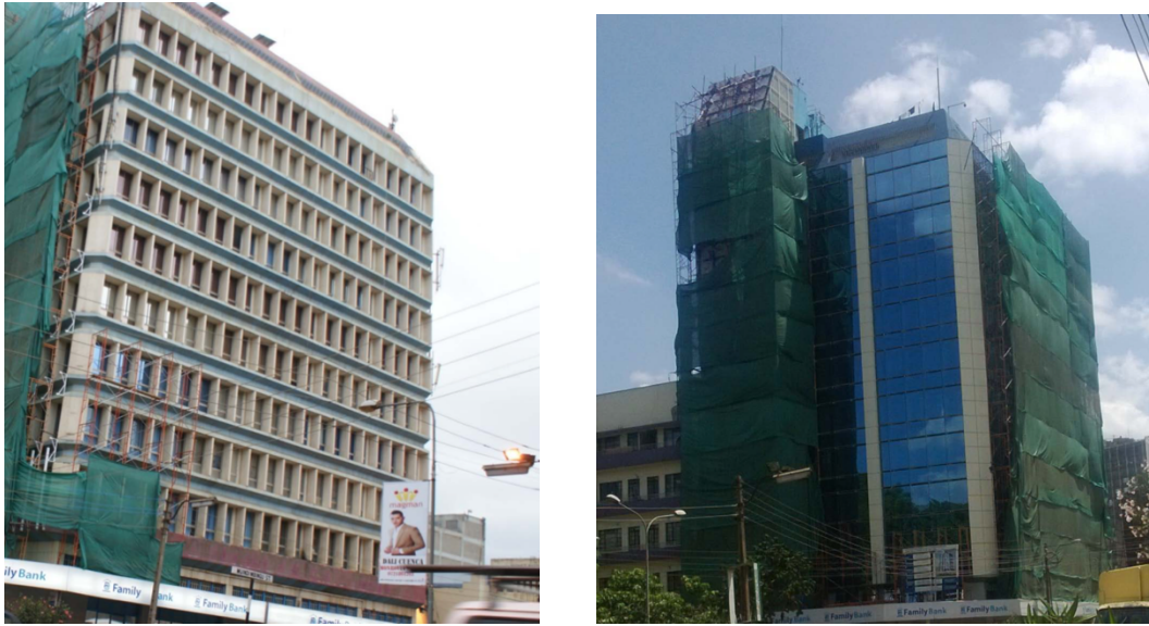
Fig 2- 14: Family bank headquarters on Muindi Mbingu street, Nairobi currently being glass cladded (2014 - 2015) Source: Musau Kimeu, July 2015
