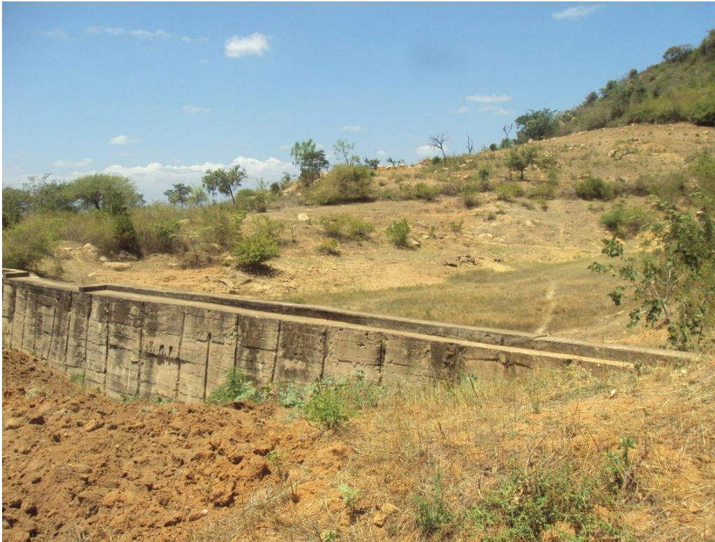
(Note the cultivated areas on the lower and upper part of the dam)
