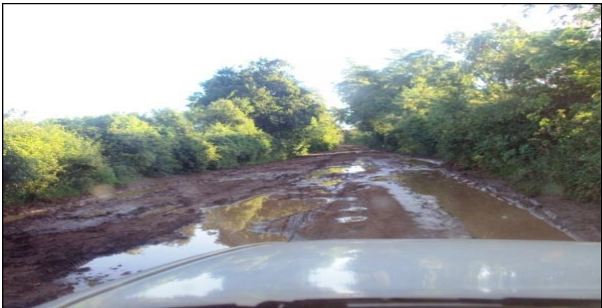
Plate 1: Dilapidated Sections of an Access Road in Kamwimbi village
