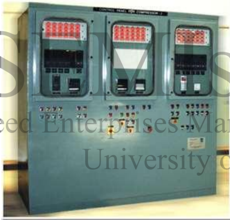
Control panel used in the processing plant
