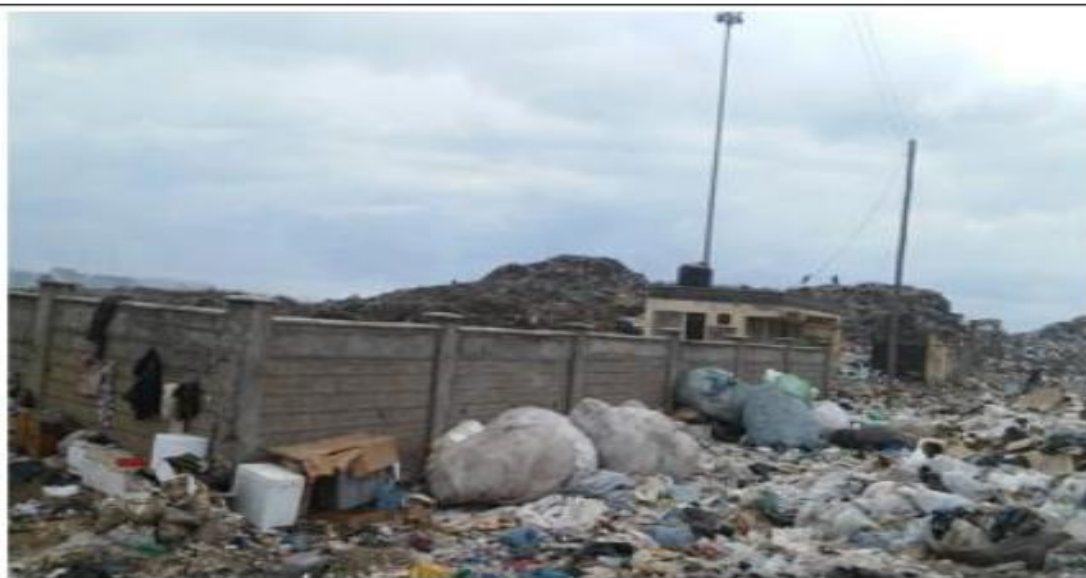
Part of the perimeter wall, only 200 metres has been constructed so far, to meet NEMA ten minimum requirements of a good landfill, to control dumping and spread of waste outside.
