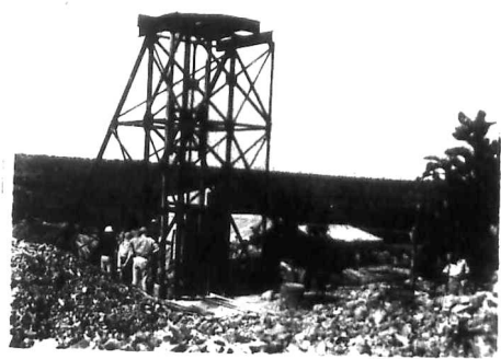
N.B. No timber is used in this shaft only steel and concrete.
