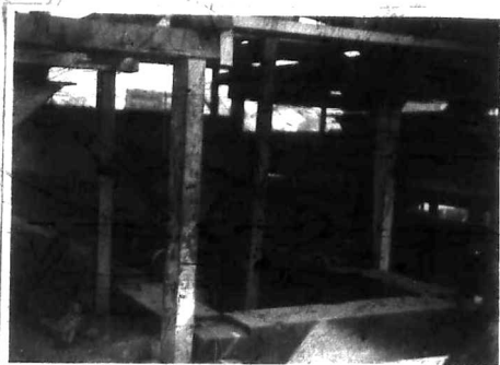
Detail of Main Shaft showing style of timber used. The cost of sinking this shaft is about $2.50 per foot. The Wacheche holdings are of no value at
