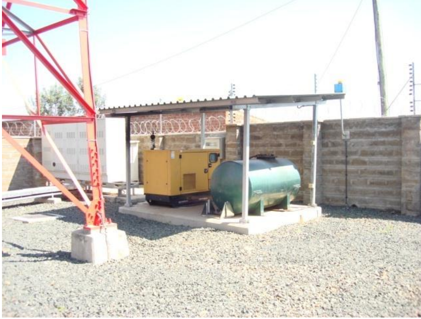
Figure 2.5: Typical Outdoor BTS Site on grid with generator
