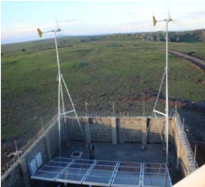
Figure 2.4 Typical Site on Hybrid Power (Combined Solar-Wind and Genset)
