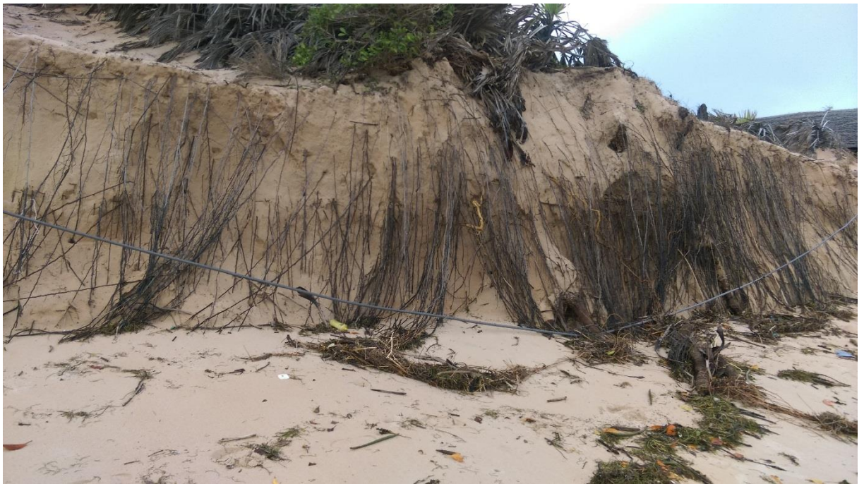
Erosion as result of wave action
