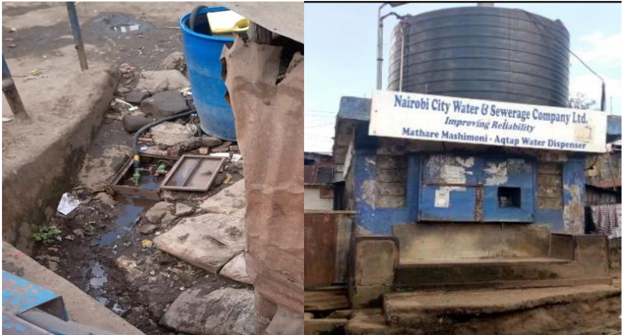
Suspected illegal connections and abandoned water network
