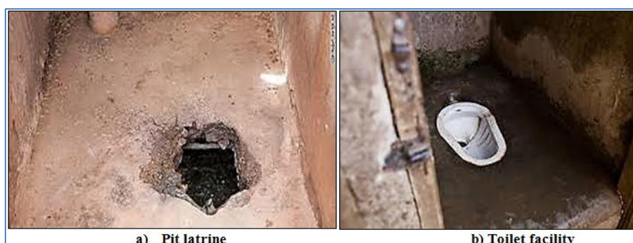
Fig-5: A photograph showing type of toilet facility in the study area
