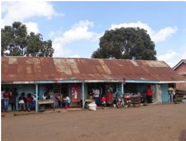
Figure 38: Decayed commercial areas
