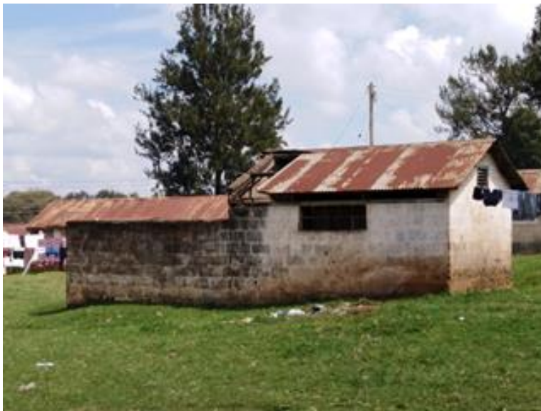
Figure 32: Degraded shared sanitary facilities.
