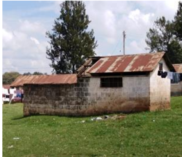
Figure 27: Dilapidated shared sanitary facilities
