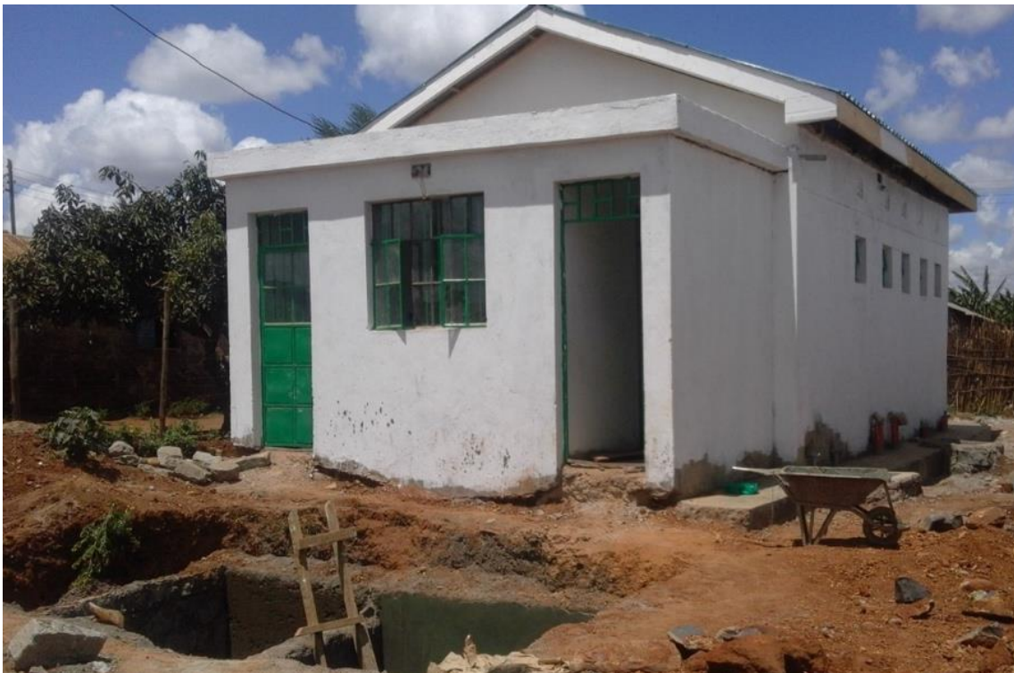
Figure.4.9. Incomplete ablution block in Munyaka settlement. Source: Fieldwork, 2016
