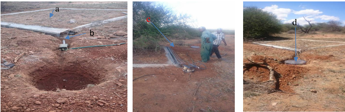
Figure 4. 1 Runoff plots a] runoff plot b] drainpipe c] construction of the runoff plots d] water tank
