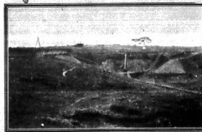
Construction work at the Nile Railway Bridge. Photo: R. H. Hubbard, Cairo.
