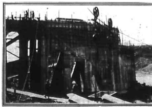
Work on the road and rail bridge over the Nile near Juba is progressing rapidly. A view of the massive concrete structure.
