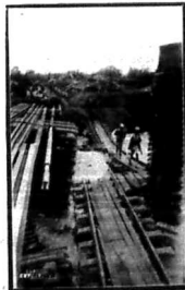
Discharge at Gode Gode. On right the original railway bridge which collapsed and on left the temporary structure still under way. Photo: J. F. P. Lobo, K.M.
