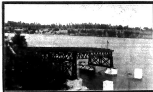
Foot steps on the construction of the Nyali Bridge which is being built by private enterprise at Mombasa and will open up the Nyali residential estate on the mainland.
