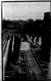
Damage at Gode Gode. On right the original railway bridge which collapsed and on left the temporary structure now being built. Photo: J. P. P. S. S. S.
