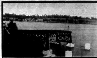
Steel girders in the construction of the Nyali Bridge which is being built by private enterprise at Mombasa and will open up the Nyali residential estate on the mainland.
