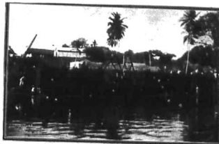
The Nyasa Bridge, Mombasa. Building sections of the structure in Mombasa harbour. Photo: E. F. Meyer.
