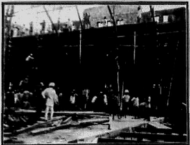
Building operations at the new Nevada headquarters of the Standard Bank of S.A., South Africa. Photo: P. H. Coll.
