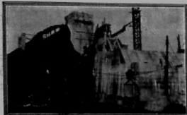
The East abutment of the bridge over the Nile now in course of construction.
