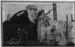
The East abutment of the bridge over the Nile now in process of construction.
