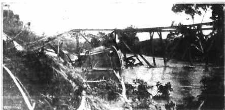
A VIEW OF THE DESTROYED BRIDGE AT KOROWO.
