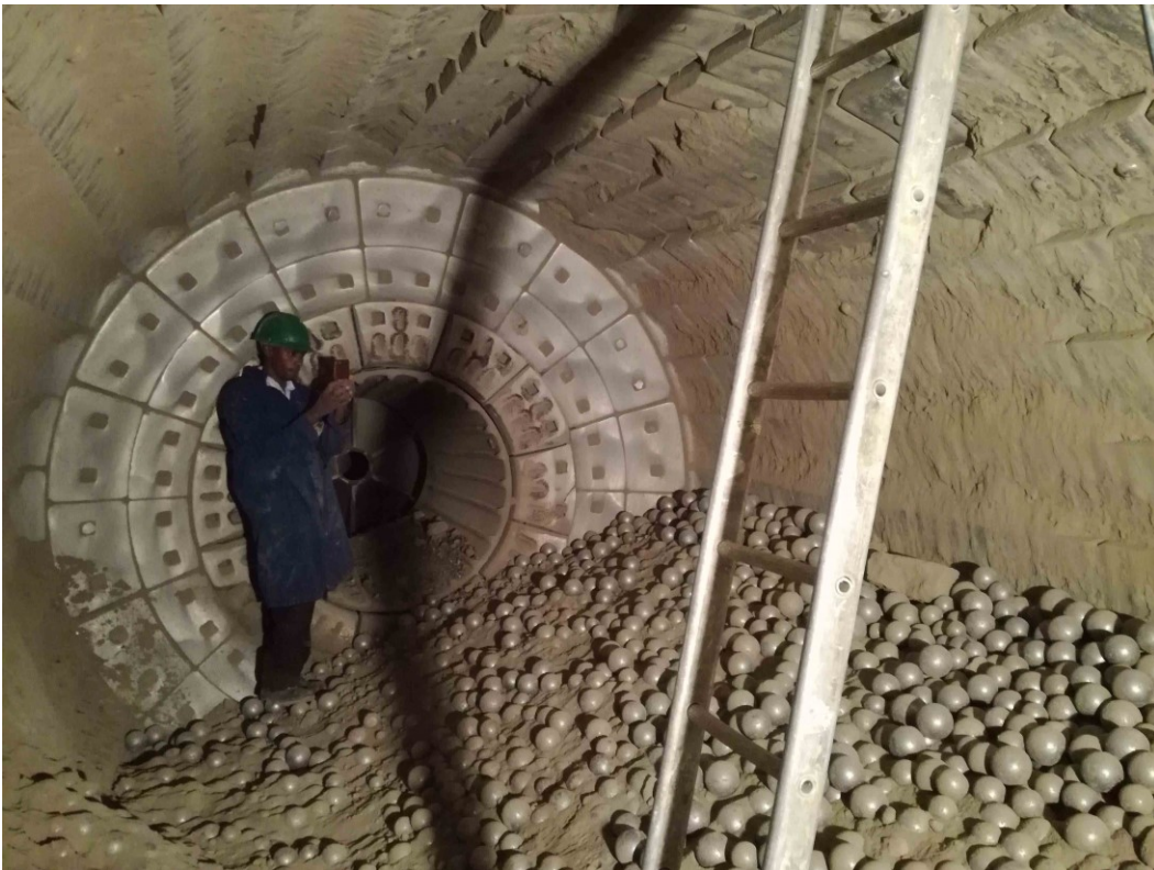
Figure 3.8: The interior of the second chamber of the clinker ball mill
