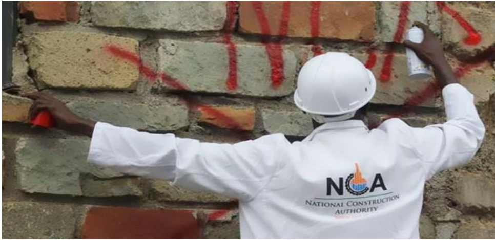
Figure 1.0: NCA Official Marking The Red “X” On A Building, Source: Construction Kenya
