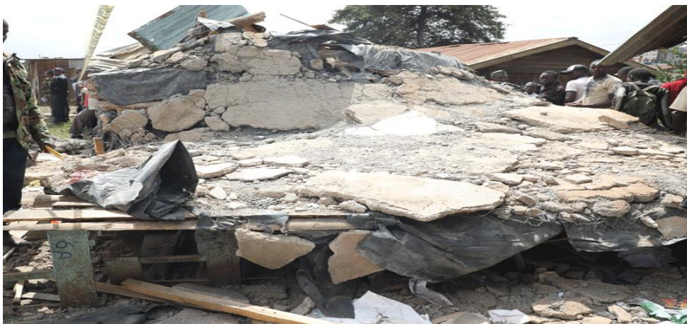
Figure 1.1: Collapsed Classroom at Precious Talents Top School, Nairobi; Source: People Daily Online, 2019
