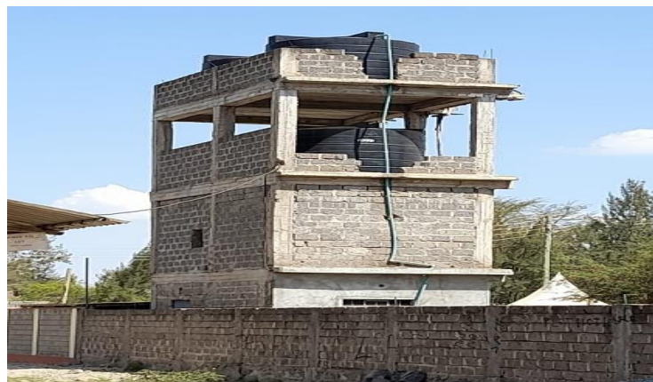
Figure 16: Overhead water tanks
