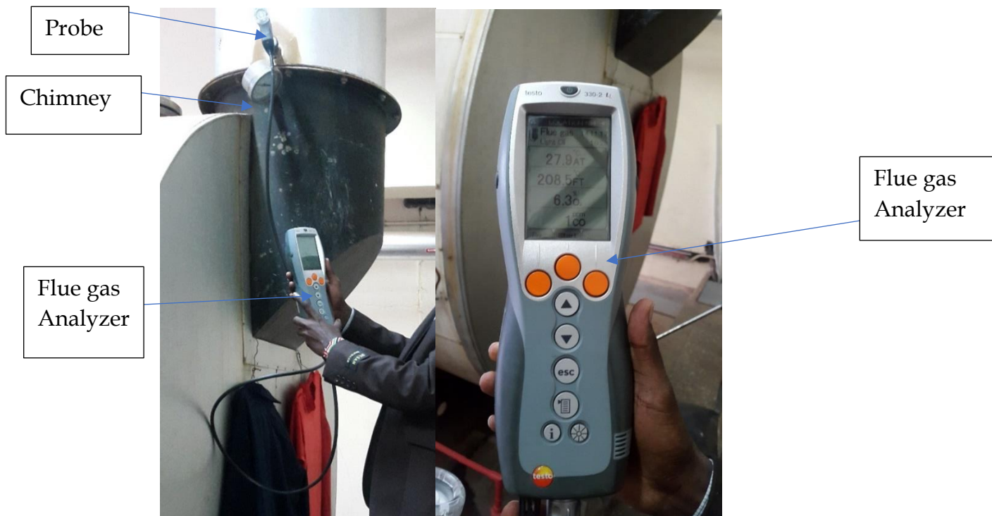
Figure 3-7- The flue gas analyzer set up to take a sample of flue gas from the boiler chimney
