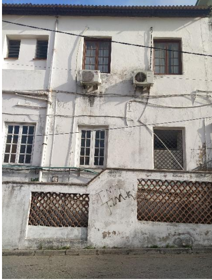
ACs on Building Walls
