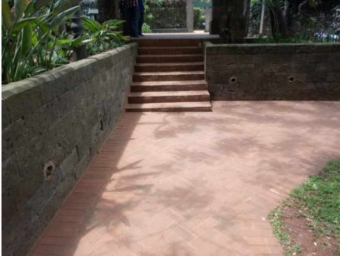
Figure 28: Steps in the Bomb Blast Park heading towards the museum (Source; Author, 2022)
