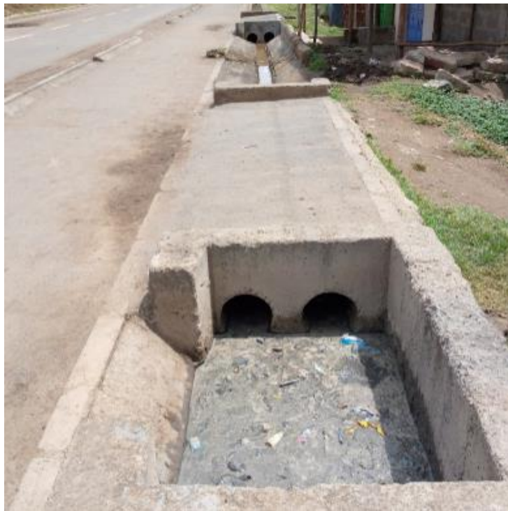
Photo 5.9: Clogged Open Drain in Ruai
