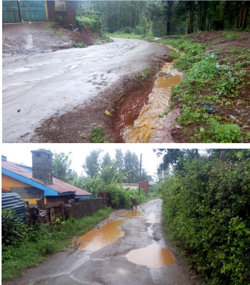
Plate 5: Existing drainage channel in poor condition
