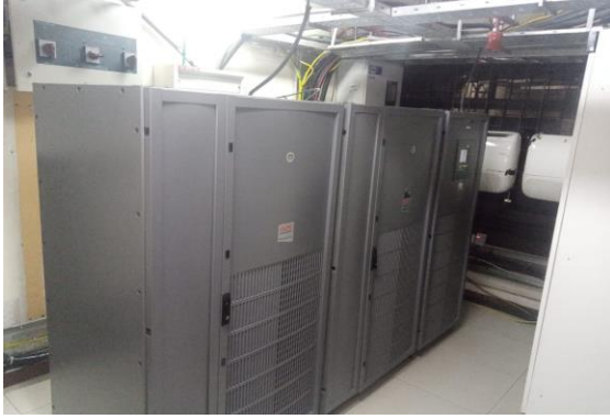
Figure 3. 1: 120kVA UPS at Power Room
