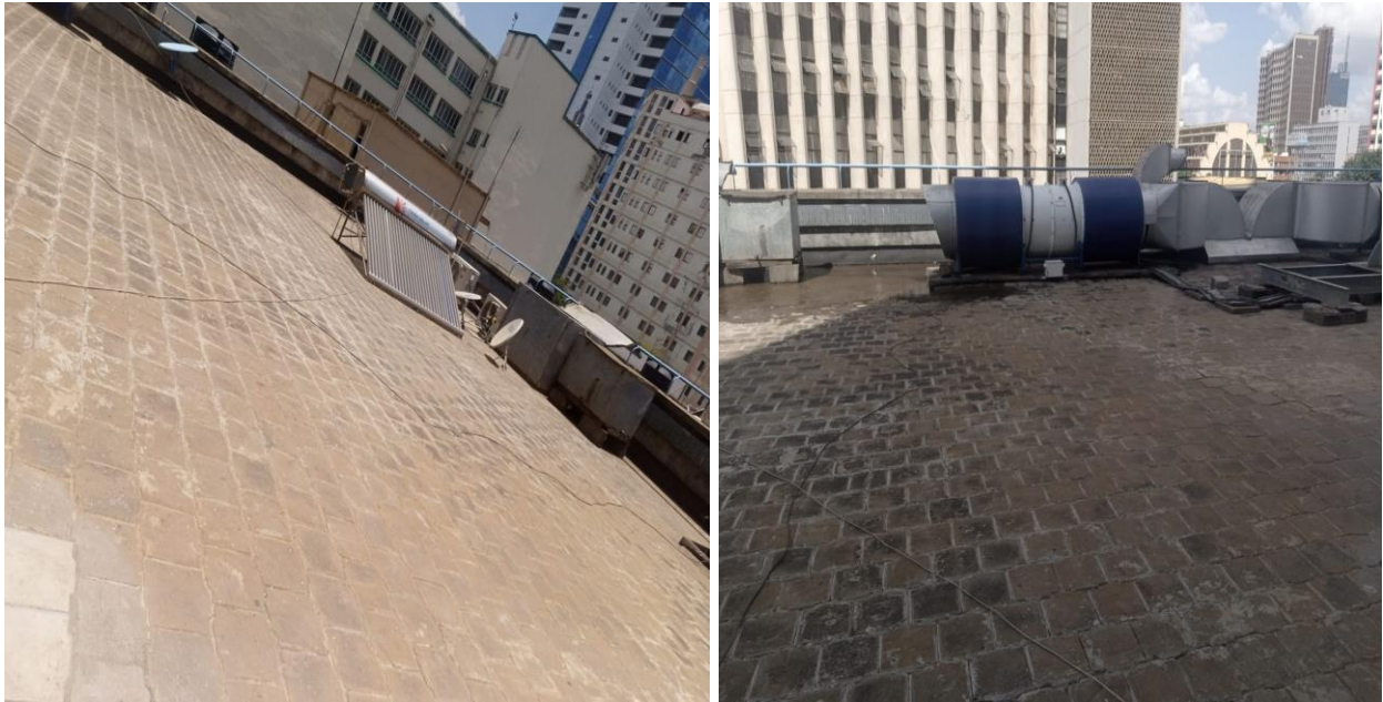
Figure 4. 27: Terrace Space for Solar PV System at Wananchi Group (K) Ltd Data Centre
