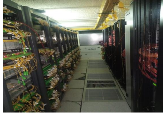
Figure 3. 2: IT Equipment Racks at the DC
