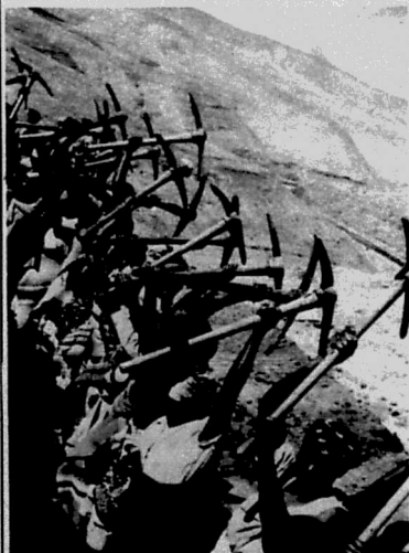
Road building in Lesotho: The effects of male labor migration weigh heavily on women
