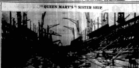
The building of the "Queen Elizabeth," sister ship to the "Queen Mary." It is going ahead at Clydebank. When completed it will be the biggest liner in the world.
