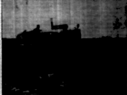
A 240 h.p. Heavy Crawler Tractor at work on a Dam Building project.
