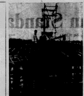
Mr. Kild (right), with his colleagues, Mr. Ben Wilson, an installation supervising engineer, on top of the International Building site, looking down on the air-conditioning ductwork.
