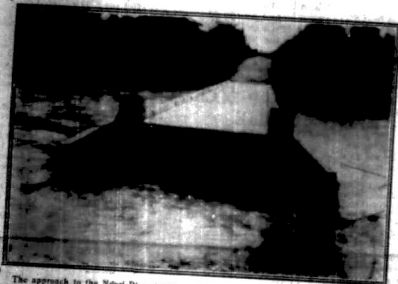
The approach to the Ngere River bridge - washed away as a result of torrential rains.
