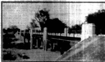
The Wamal Bridge of 5 spans with a total length of 183 feet 6 inches on the Morogoro-Tuziani Road.
