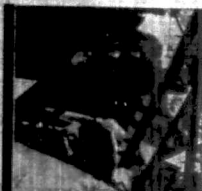
Conveyor feed from secondary crusher to bucket elevator
