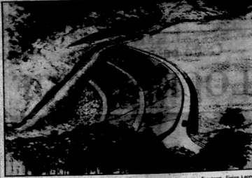
WORK is in progress on the construction of the Gunge Valley Dam, near Freetown, Sierra Leone...
