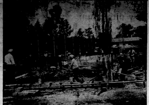
Construction under way on the new £200,000 municipal hall and offices for Nakuru Municipal Council. The new block on the southern side of the present hall and the street should be completed before the end of the year.
