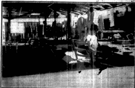
One of the dormitories showing that there is plenty of room and also showing the space between walls and roof where the rain gets in occasionally. (This defect is being remedied). Photo: K. Gandar Dover.
