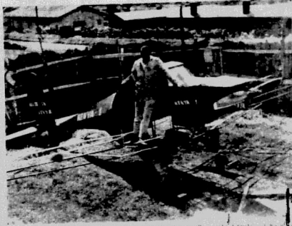
Back that will hospital. Mr. Eric Kamamba stands on the partially completed road.
