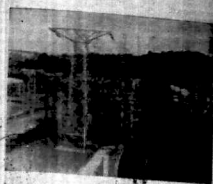
A blacktop of the switchgear transformers at the Tana Power Station near Fort Hall.
