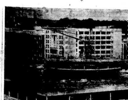
The round tower of the Nairobi Hilton Hotel, which is designed to contain 300 bedrooms, is gradually taking shape. More towers in use from the top of a 200-foot tower. Below it are the three rectangular towers which will be public rooms, shops and offices.
