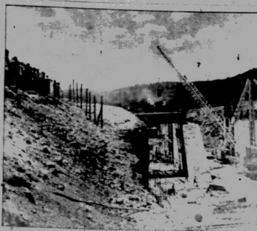
The Ministry and great work commenced in the new building of a hospital on the Tere road. The work is well advanced.
