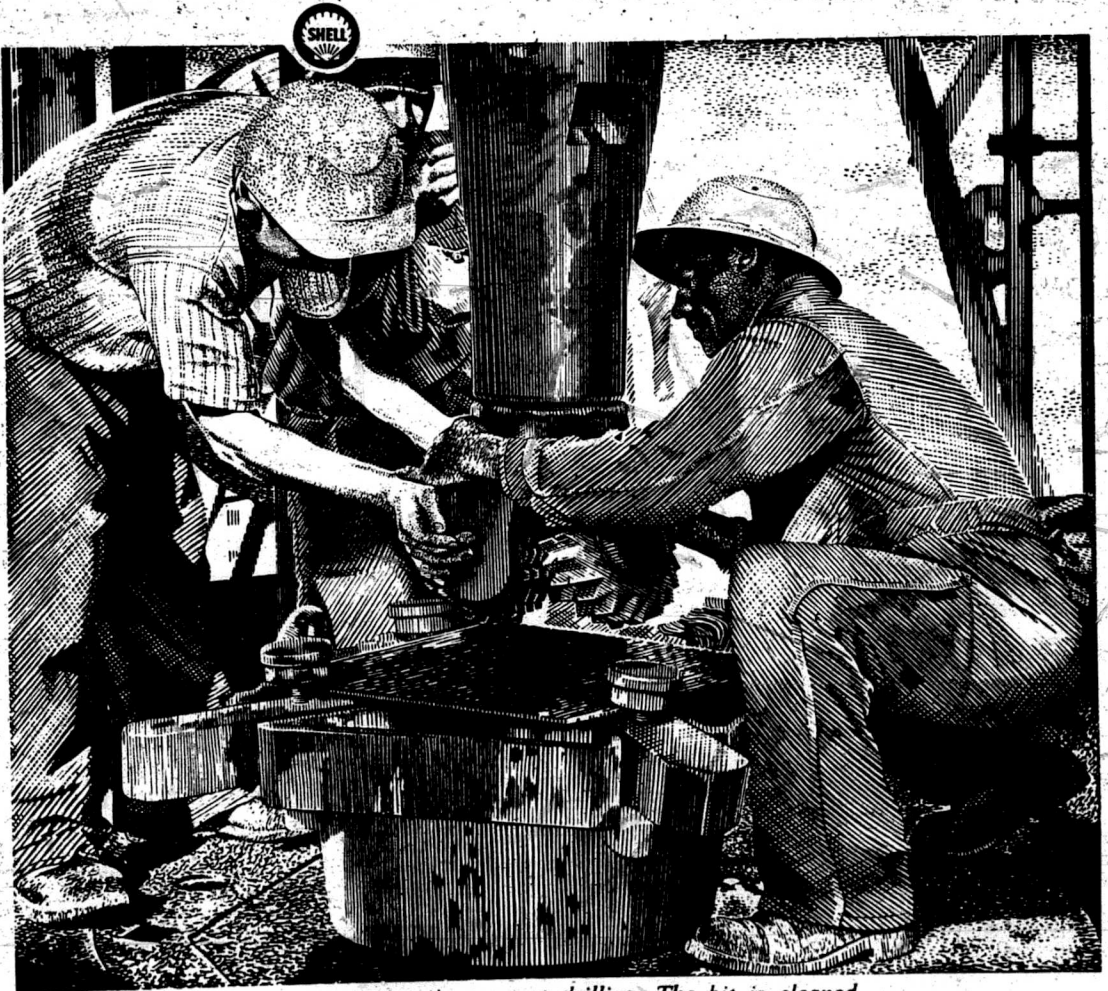
Getting ready to start drilling. The bit is cleaned and then attached to the drill pipe and screwed fast.
