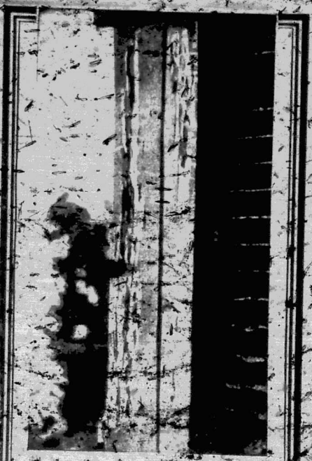
Without a lack of protection the destruction caused by White Ants was great. The picture is rendered in black in an incredibly short time.
