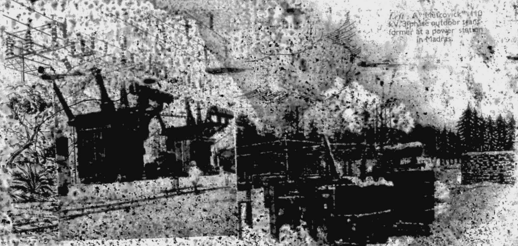
Fig. 2. A Metropolitan 11,000 V 3-phase transformer in a plant in Madras.
