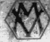
Fig. 1. A Metropolitan 110 kV 3-phase outdoor transformer at a power station in Madras.
