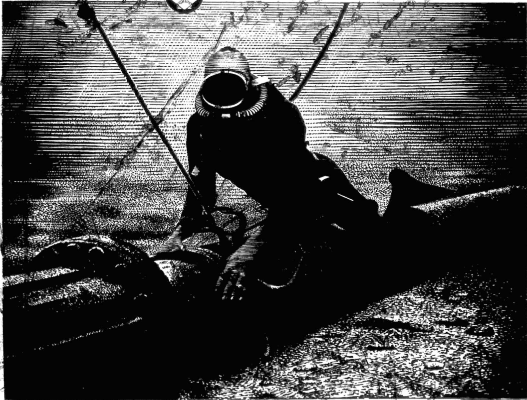
The flexible hose connections of a 16-inch diameter pipeline being inspected by a diver. This pipeline speeds the discharging and turn-round of tankers.
