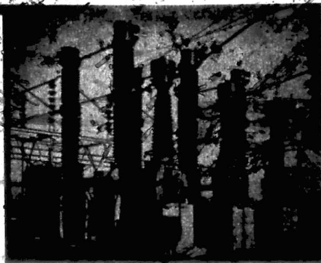
220-kV small-oil-volume circuit-breakers in Australia
