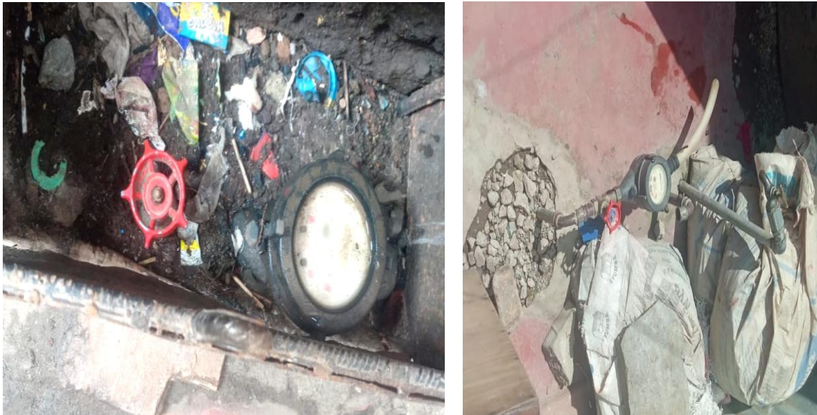
Figure. 4.14: Vandalized JM and Disconnected JM respectively at Soweto Kayole (SK)
